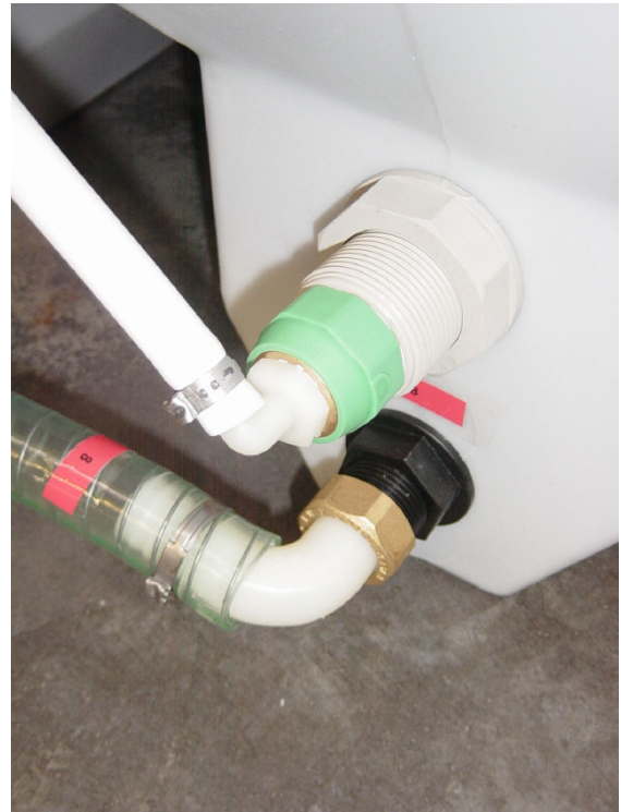
Connection aerator unit
