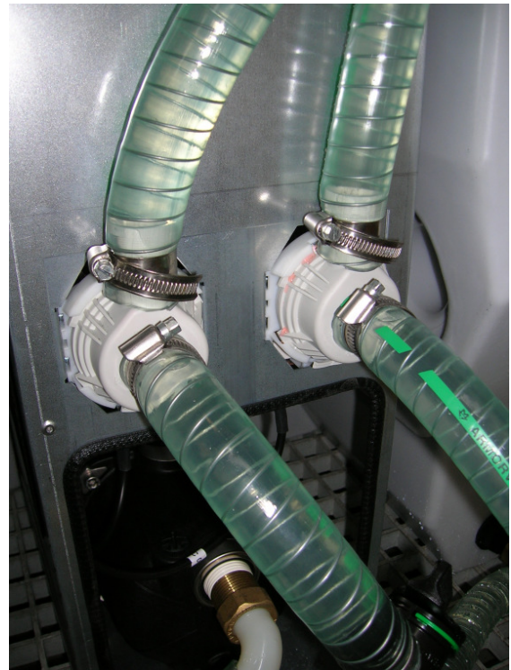
Suction lines + pressure lines
